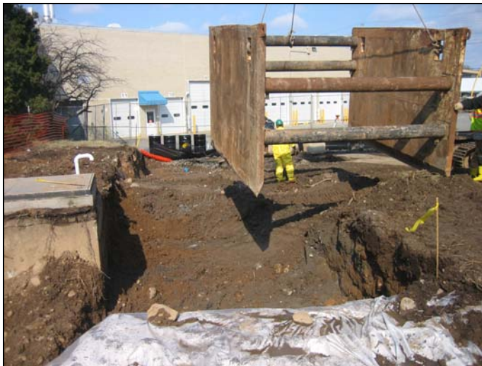
Following cleanup of PCB-contaminated soils, a trench box is lowered to facilitate removal of buried relic industrial wastewater septic tanks.
